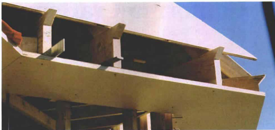
Supporting the main cornice. Triangular trusses made of Douglas-fir 2x4s fan out from the wall framing to serve as backing for the cornice roof and soffit. The trusses are held in the same plane by plywood gussets. The beaks on the bottom cords of the trusses anchor the crown molding.
